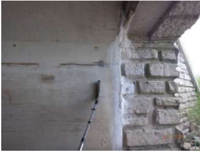
Figure 20. Leakage and efflorescent staining at northwest corner.
