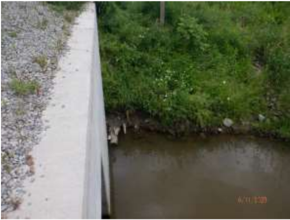
Figure 29. Erosion at southeast corner.
