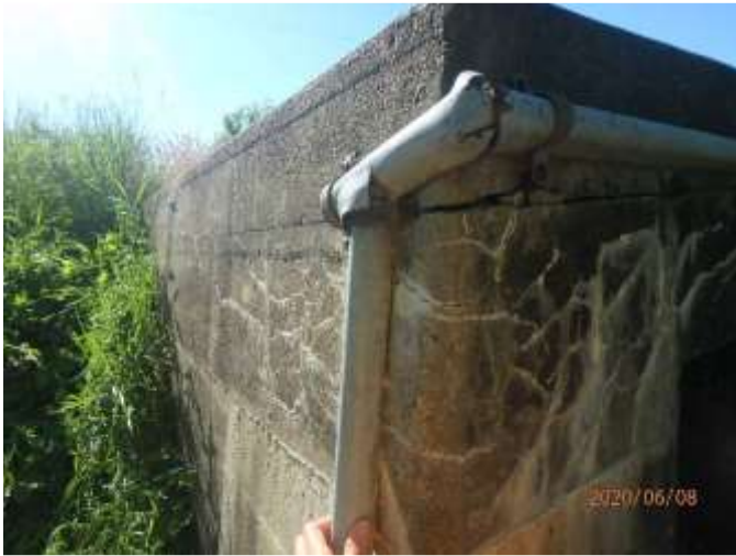
Figure 16. Wide horizontal crack at south east corner.
